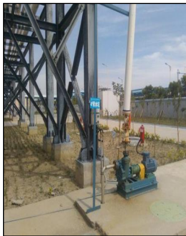
4.2-10 储罐区打料泵
