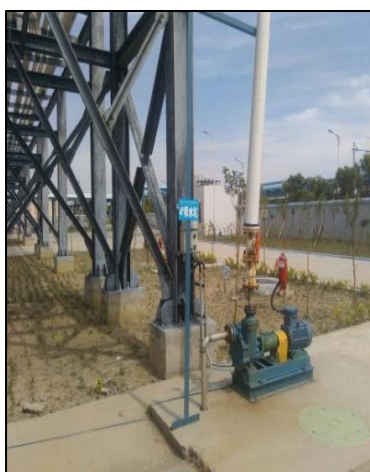
4.2-10 储罐区打料泵
